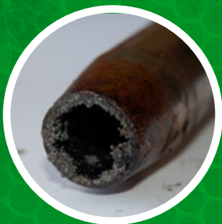
WITHOUT PROTECTION, AFTER WELDING
